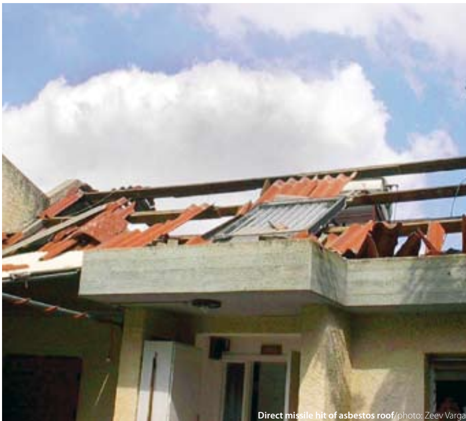
Direct missile hit of asbestos roof/photo: Zeev Varga
